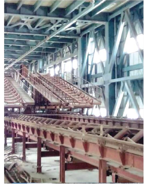
COAL HANDLING PLANT AT BHEL, BARAUNI
