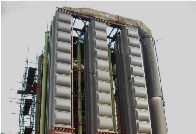
PRIMARY GAS COOLER & GAS PRE-COOLER, SAIL - ROURKELA STEEL PLANT
