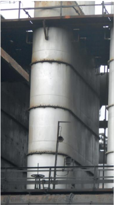
PRIMARY GAS COOLER
