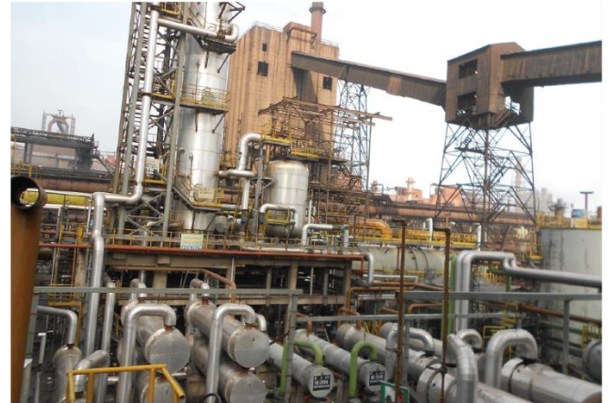
BENZOL ABSORPTION & DISTILLATION PLANT AT SAIL - DURGAPUR
