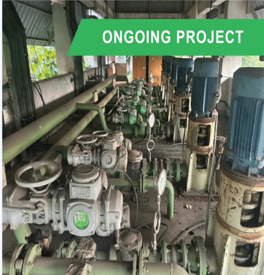
DVC – BOKARO (PRE TREATMENT AND ETP PLANT)
