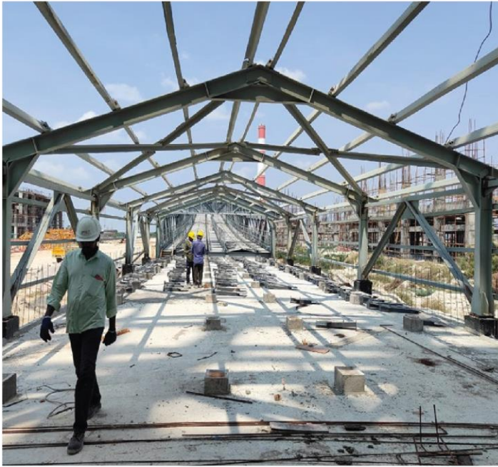
UDANGUDI SUPER CRITICAL THERMAL POWER
