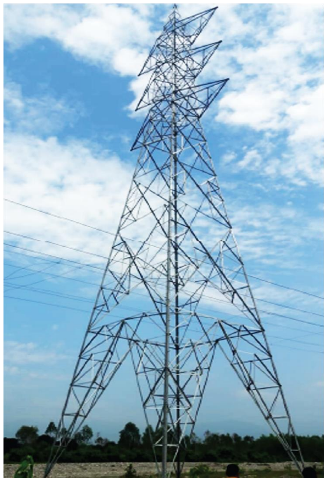
132 KV D/C TRANSMISSION LINE FROM RANIKHET TO BAGESWAR - (LINE LENGTH - 43 KM) CLIENT - PTCUL, UTTARA- KHAND
