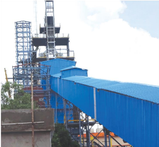
BELT CONVEYOR SYSTEM FOR TRANSPORTATION OF CALCINED DOLOMITE AT SAIL- DSP
