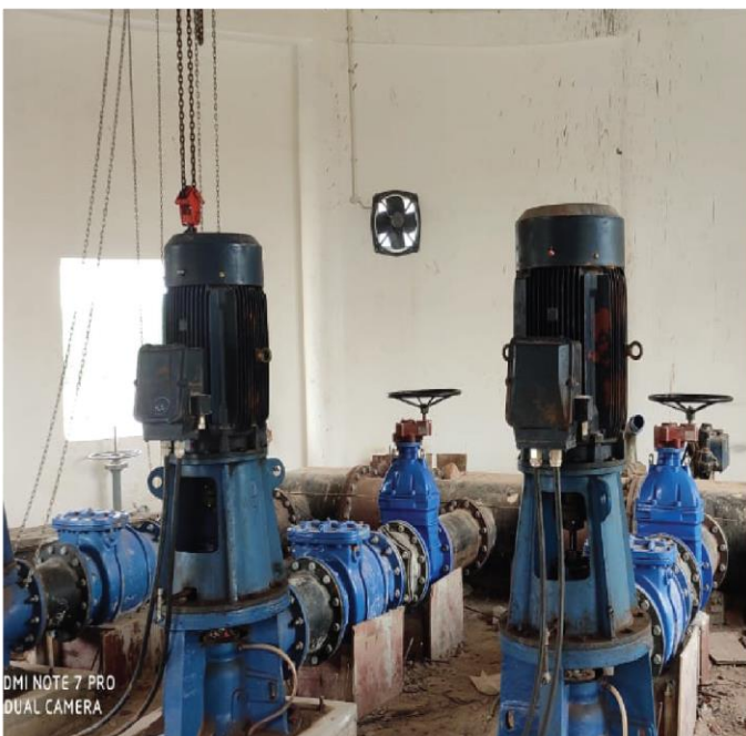
INTAKE PUMP HOUSE WITH VERTICAL PUMP
