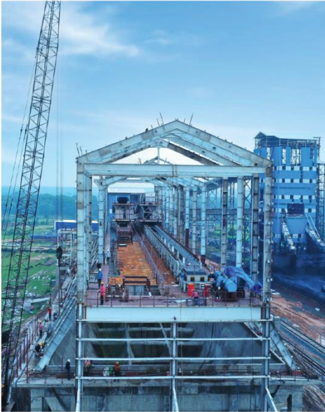
COAL HANDLING PLANT AT PAKRI
